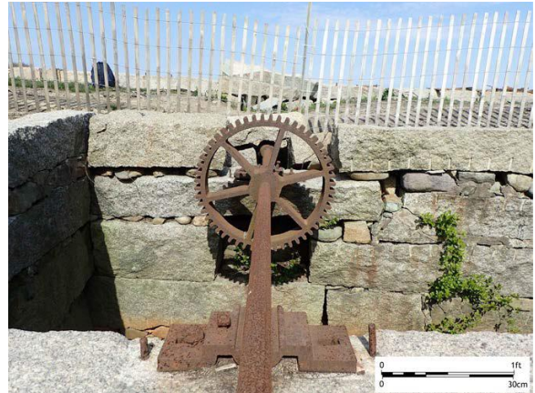
FIGURE 7: PINION GEAR, SHAFT AND BEARING TO POWER LINE SHAFT IN LOWER YARD (PAL PHOTO)
