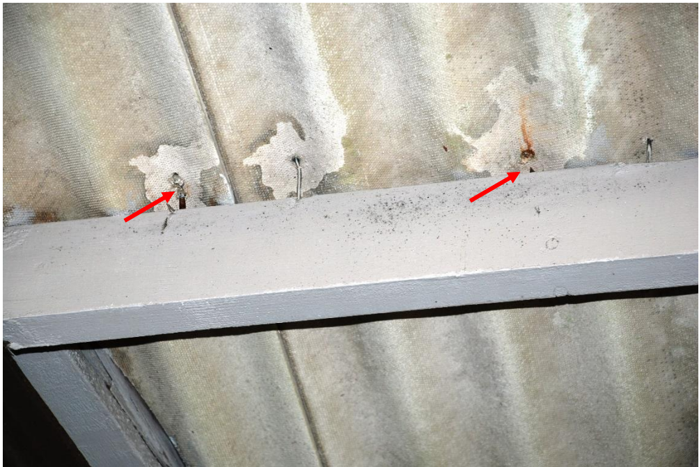
Photo 7 - View of roof fasteners at underside of deck. Note: corroded and broken fasteners.
