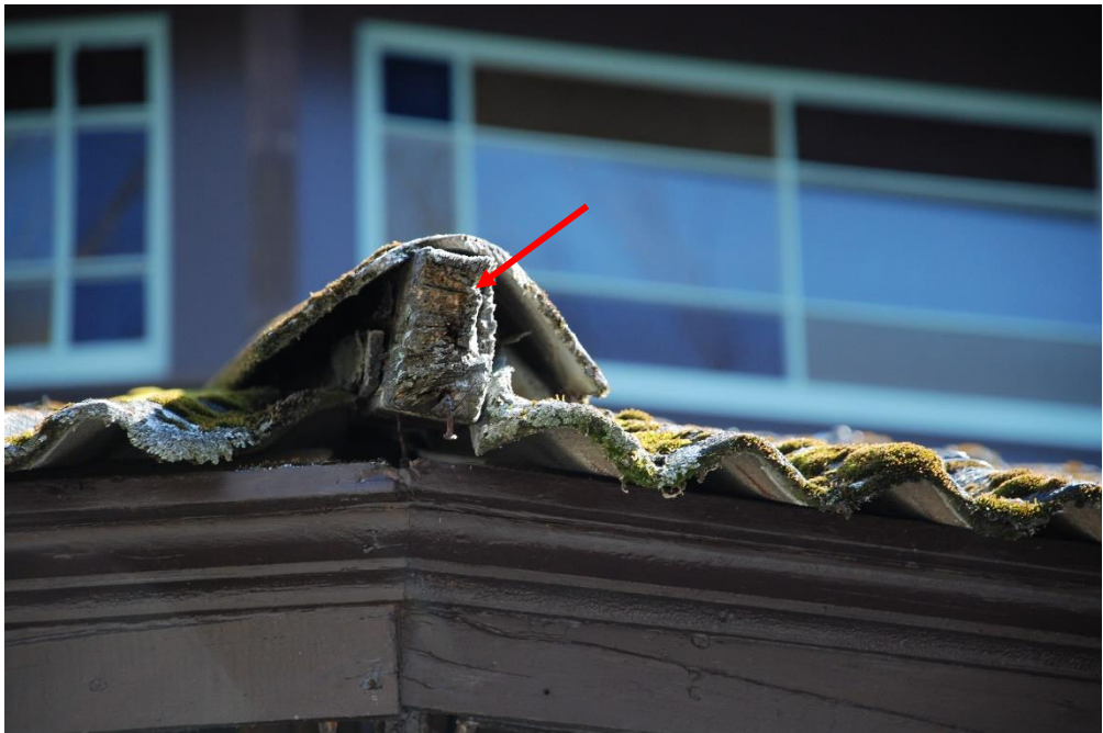
Photo 15 - View of missing wood fascia block at hip. Note: rotted hip pole.
