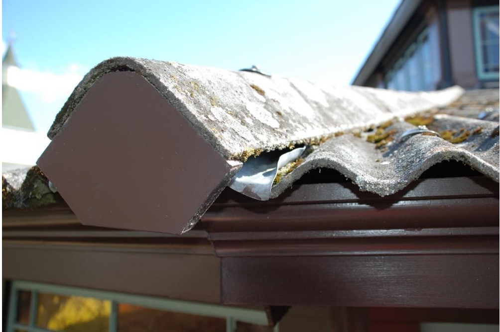
Photo 14 - View of wood fascia block at hip.
