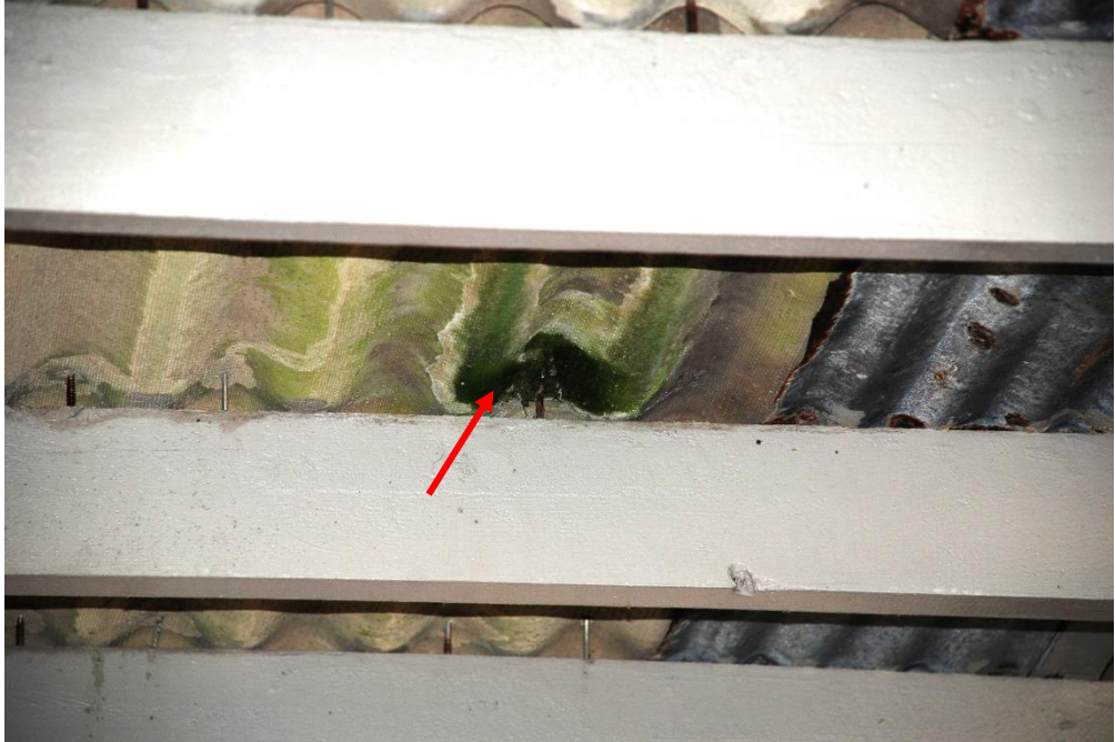
Photo 8 - View of underside of roof at apparent leak location. Note: algae growth.
