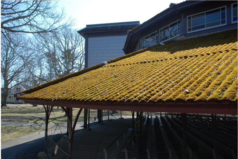
Photo 25 - View of moss covering lower roof at northeast corner.
