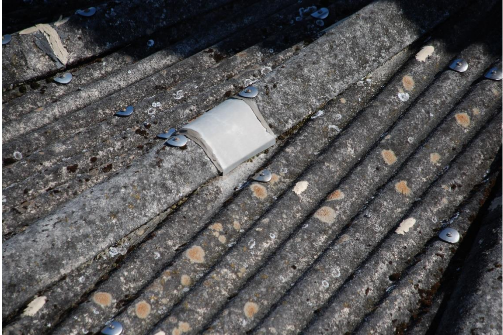
Photo 19 - View of sheet metal patch at hip cover.
