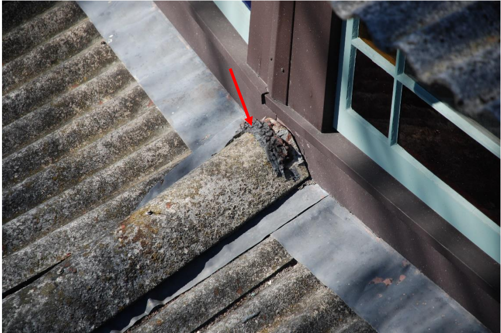
Photo 17 - View of uphill end of hip cover. Note: old black sealant residue.
