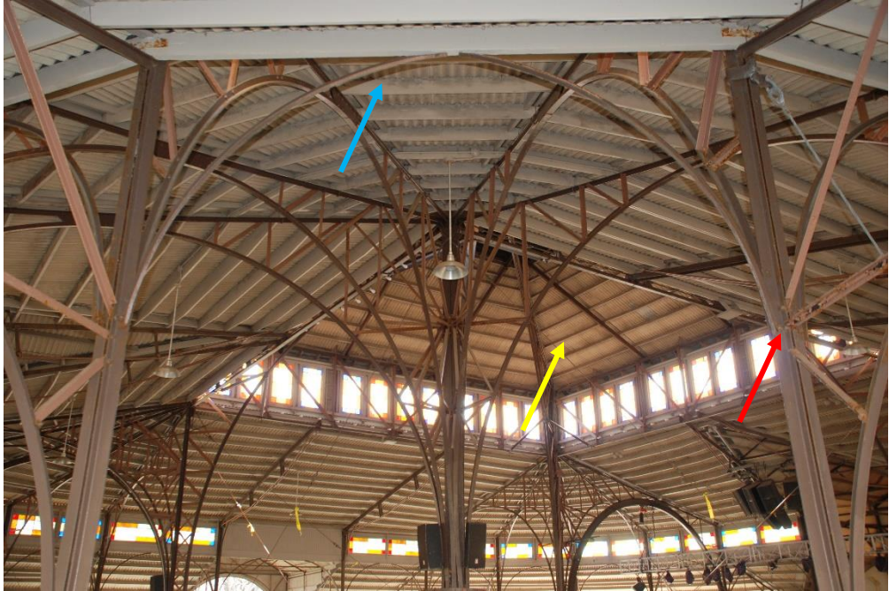
Photo 3 - Interior view of roof structure. Note: Iron truss (red arrow), Wood purlin (blue arrow), cement asbestos roof panel (yellow arrow).
