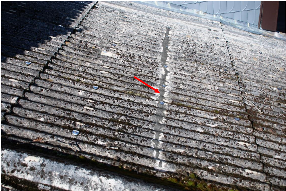
Photo 10 - View of sealed crack at exterior side of cement-asbestos panel.
