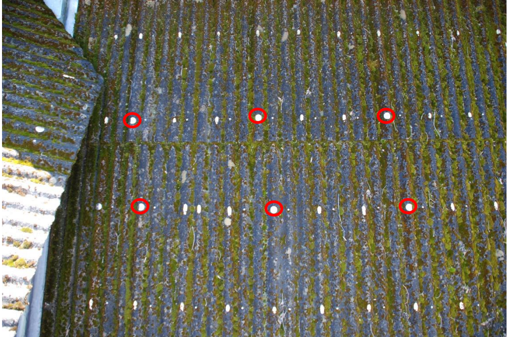
Photo 5 - View of roof fastening pattern. Note: red circles indicate new stainless steel fastener pattern.
