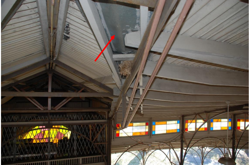
Photo 23 - View of unsupported metal valley liner at interior.
