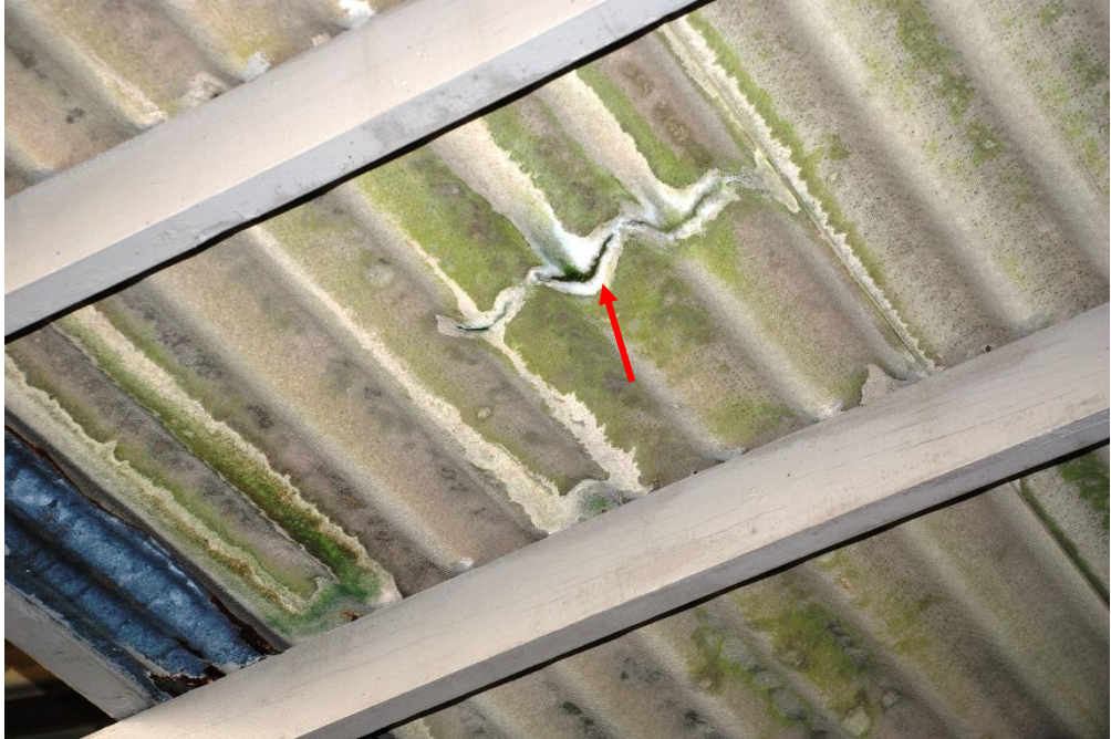
Photo 9 - View of crack at underside of cement-asbestos panel.
