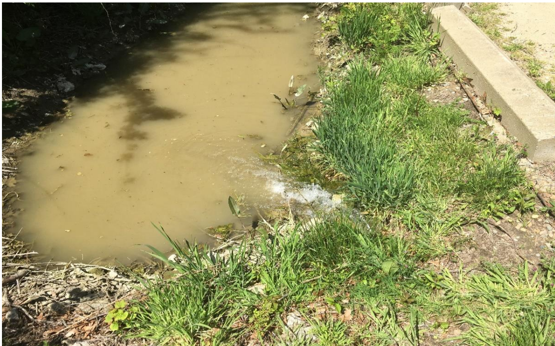
Photo 6: Small stormwater basin with sump pump discharging adjacent to parking lot.
