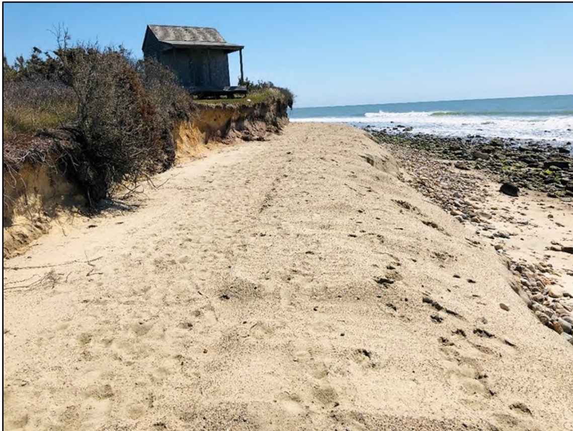
Figure 3. Photo looking east along first completed construction event for cobble berm and sand veneer – May 2020.
