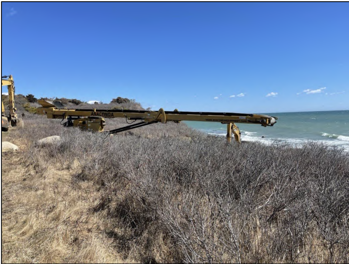
Figure 12. Photograph showing the use of a conveyor belt to transport material over the bank at 21 East Lane.
