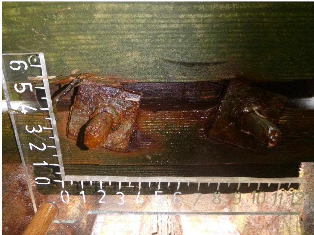
Photo 34 – The inshore deck curb connections do not go through the 4 inch by 4 inch board.
