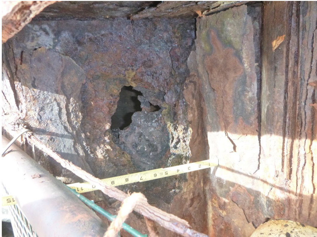
Photo 11 – Larger corrosion hole in the sheet pile web.
