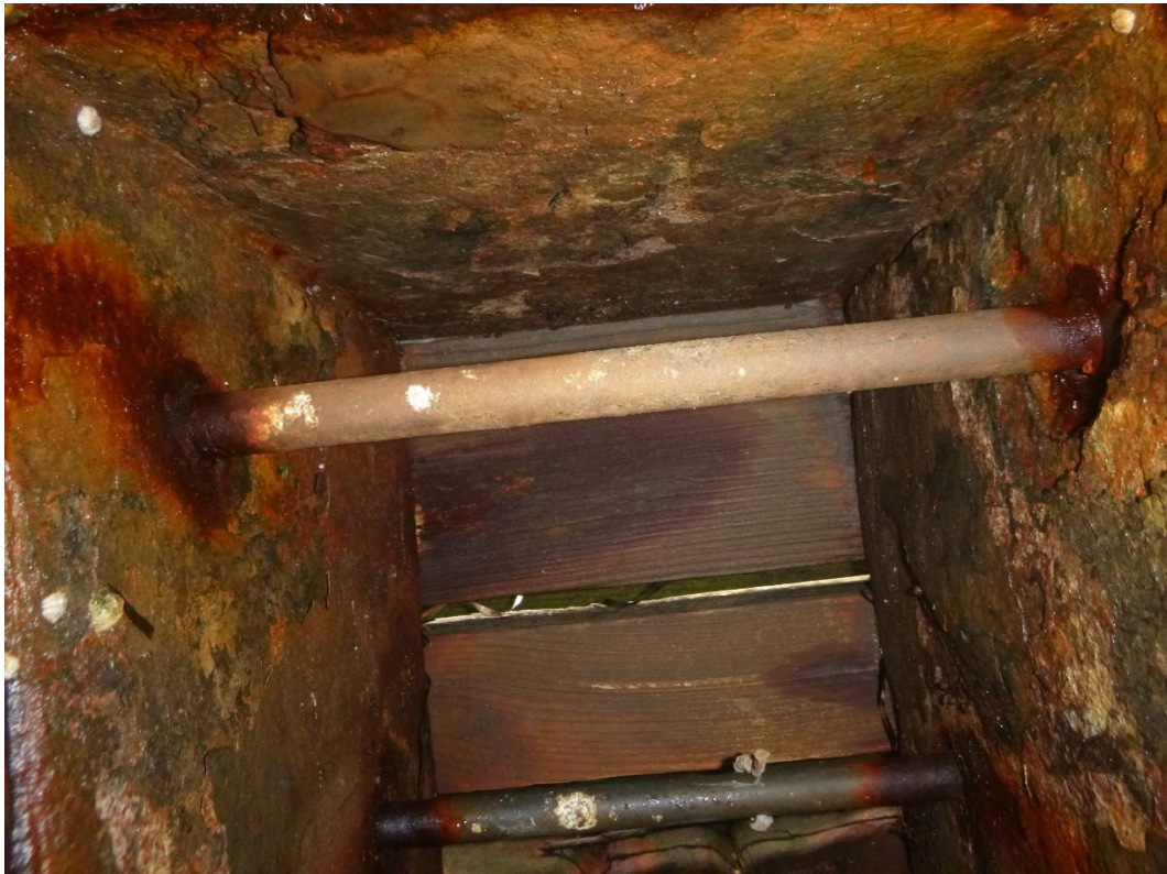
Photo 28 – Corrosion on the inside of the channel looking up.
