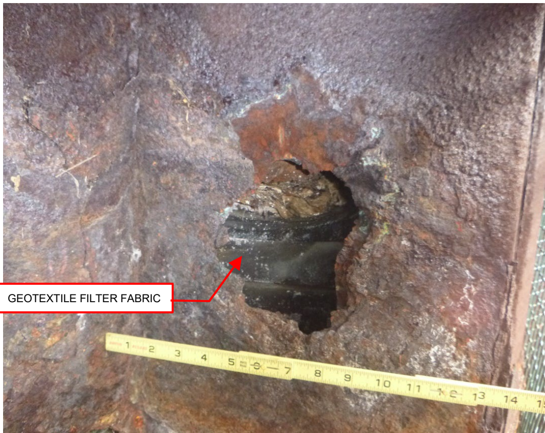
Photo 10 – Close up of corrosion hole in the sheet pile with filter fabric visible
