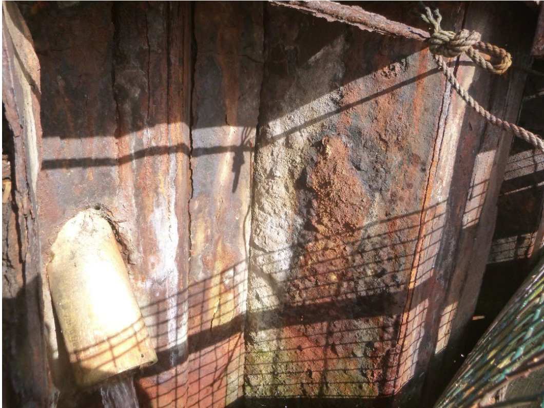
Photo 7 – Close up of the sheet pile with heavy corrosion byproduct.
