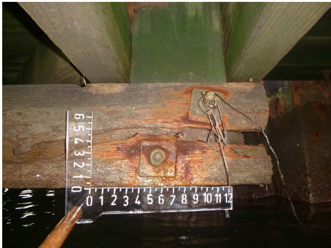
Photo 20 – Fungal decay extending into the connection between Bents 5 and 8.
