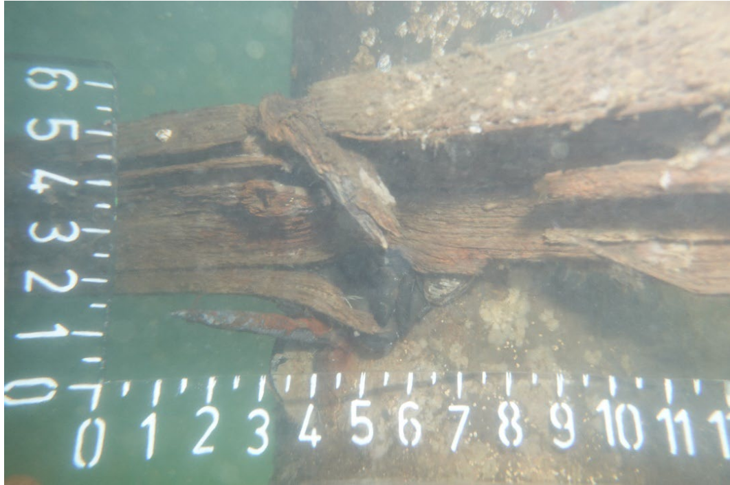
Photo 35 – Close up of the severe deterioration of the wale.
