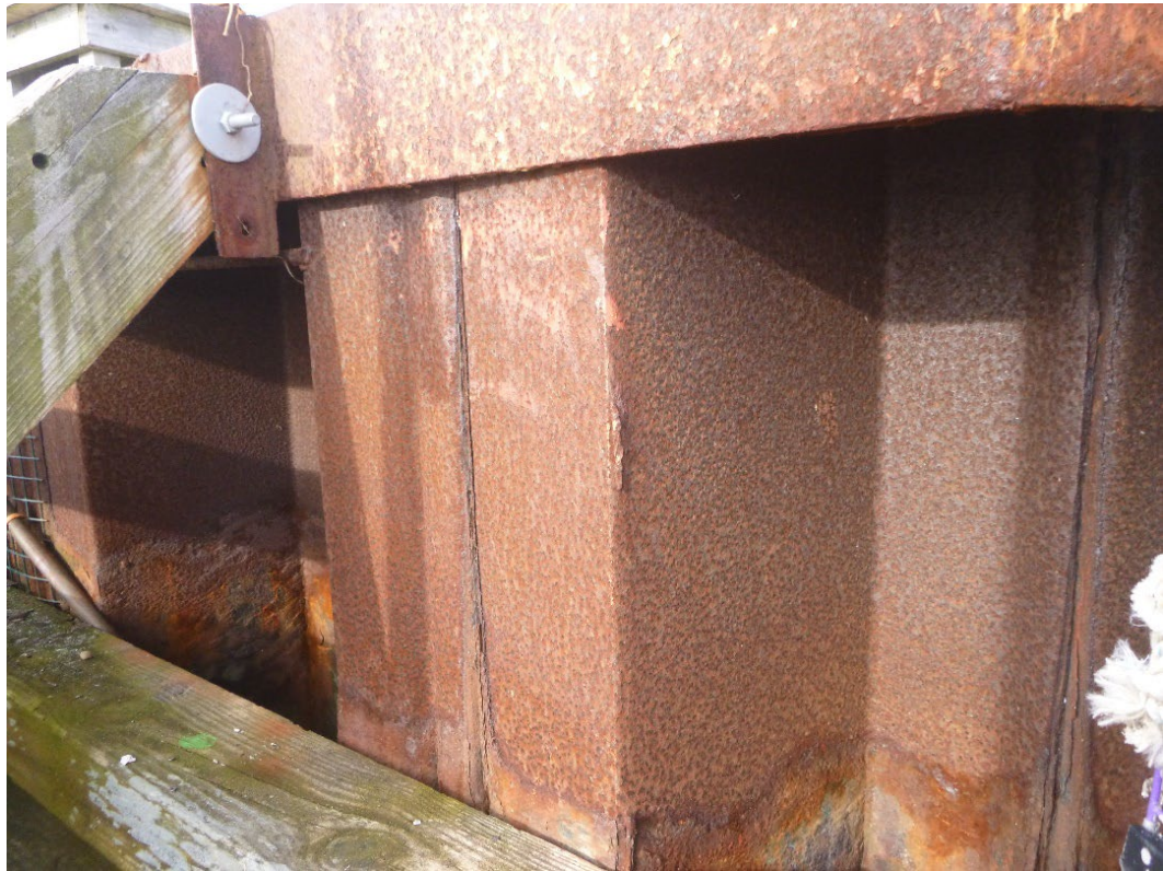
Photo 5 – Close up of typical sheet condition with surface corrosion and wavy steel.
