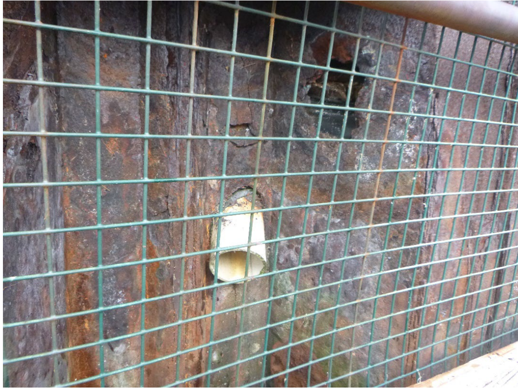
Photo 9 – Corrosion hole above an outfall pipe.
