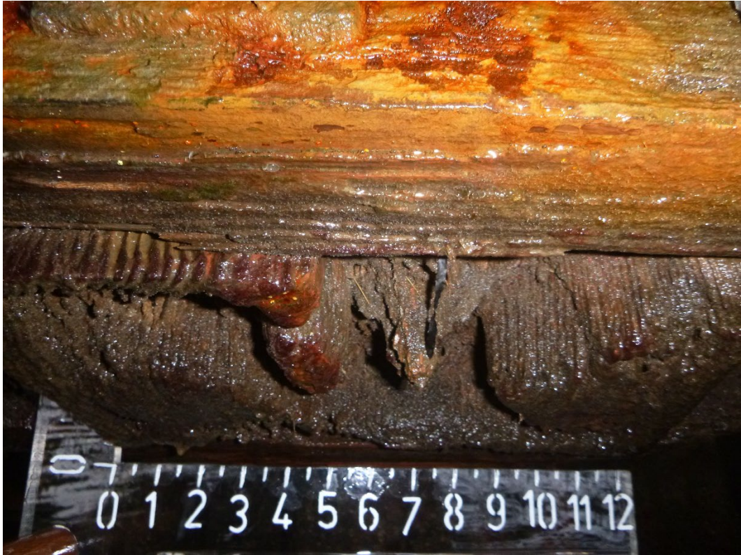
Photo 21 – Fungal decay extending into the connection between Bents 5 and 8.
