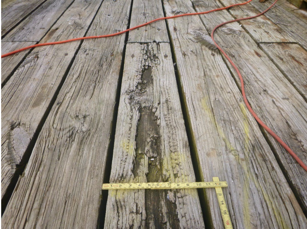
Photo 31 – Close up of the fungal decay on the timber decking.
