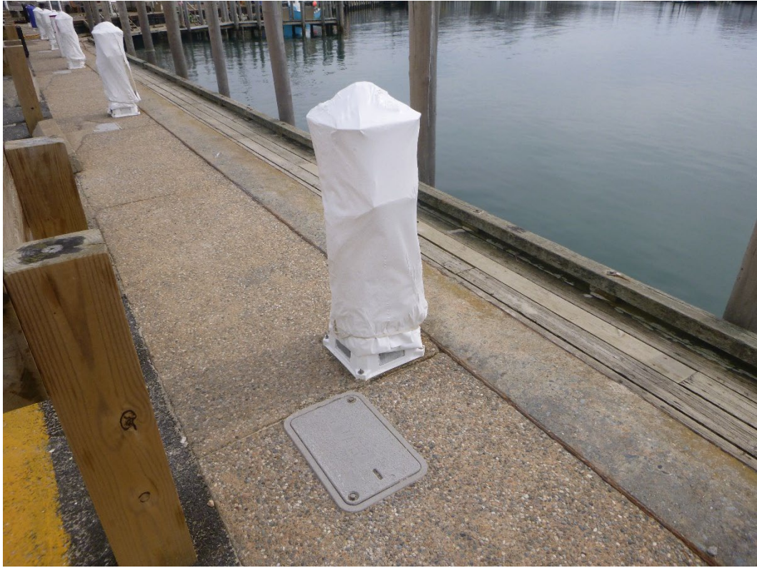
Photo 41 – Shore power pedestal.
