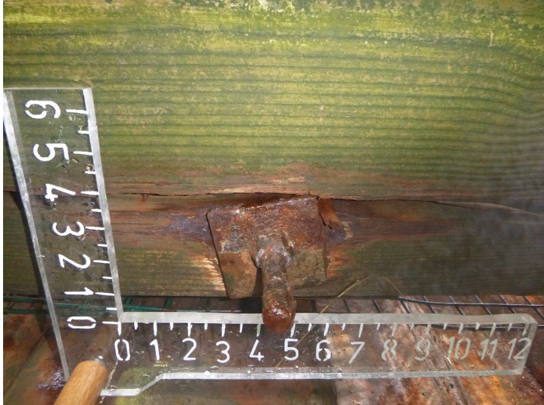
Photo 33 – Typical corrosion on the underside of the deck curb connection bolts.
