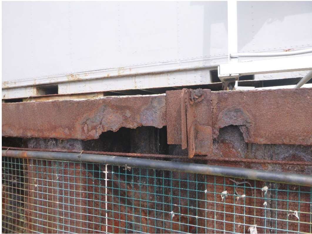
Photo 13 – Steel sheet pile cap with severe knife edging.
