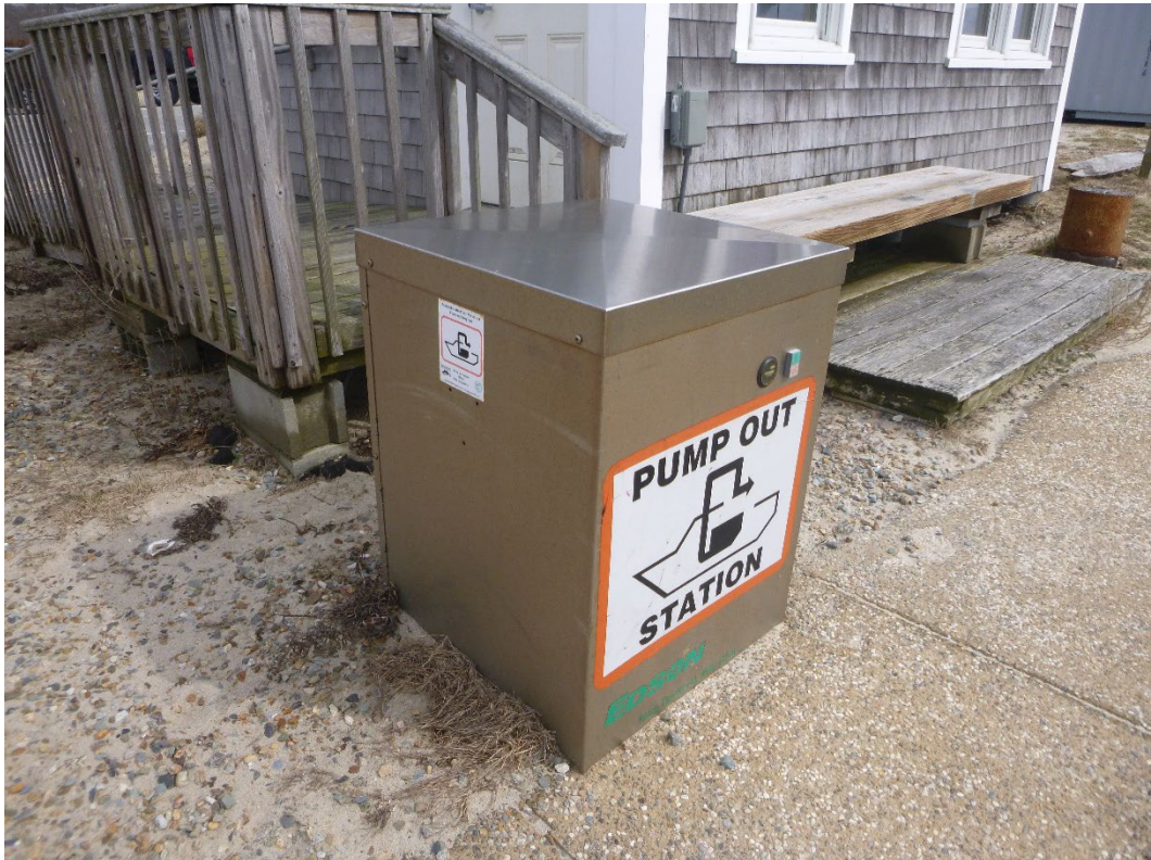
Photo 40 – Pump out station behind the bulkhead.
