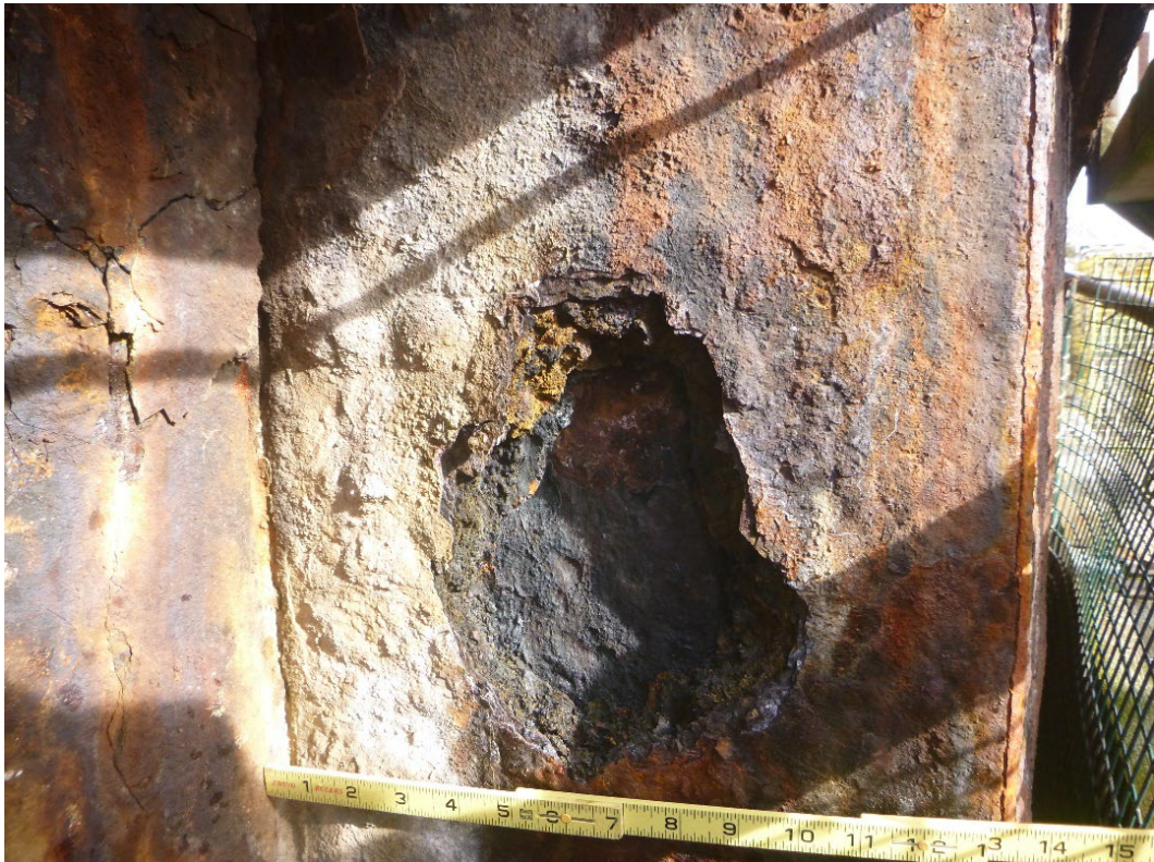
Photo 8 – Cleaned area of the sheet pile with wavy steel and heavy corrosion byproduct.
