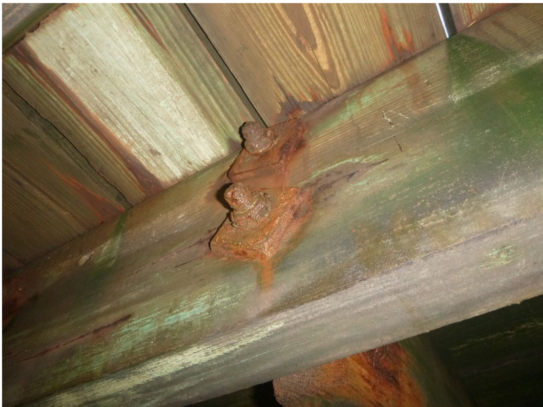
Photo 22 – Close up of the back of the butt connection between Bents 6 and 9.
