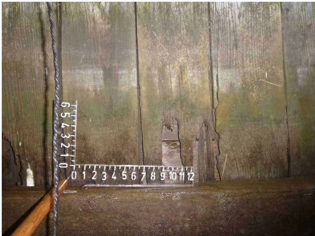
Photo 4 – Holes in the timber bulkhead in the tidal zone with new timber visible behind.
