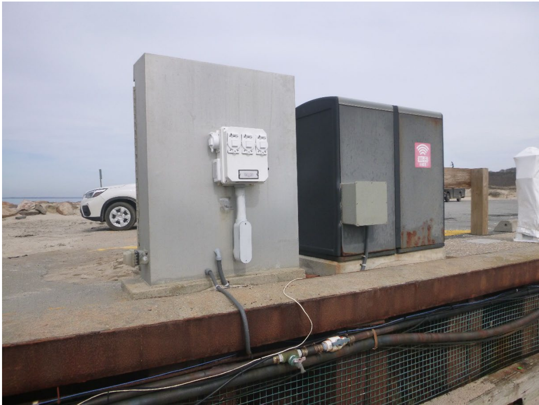
Photo 42 – Electrical transformer providing power to the floating docks.
