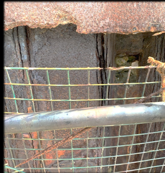
Example of visual corrosion to dock bulkhead
